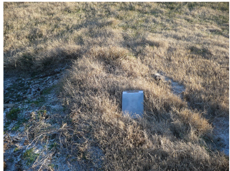
Photo #4 – depression near right wall of spillway chute near the toe
