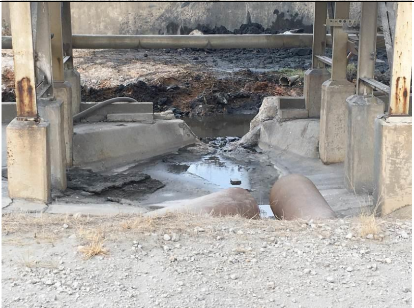
Photo # 6 View of the outlet area of the steel culverts under the conveyor system which feeds the radial arm stacker
