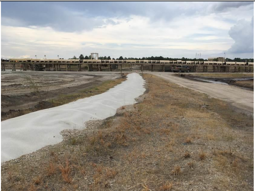
Photo # 4 View of the eastern gravel berm with a geomembrane cover facing north.
