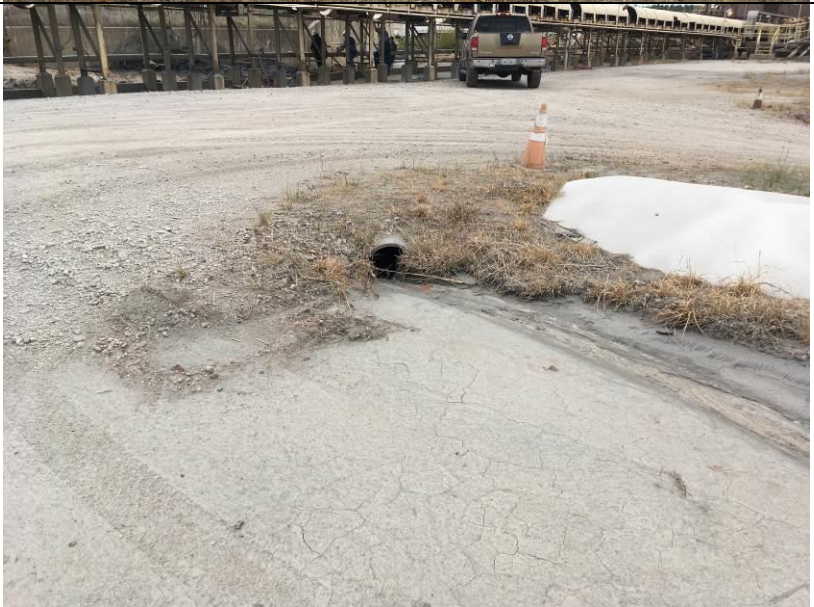
Photo # 5 View of the inlet culvert pipe that discharges water from the stackout area into the drainage ditch under the conveyor system.
