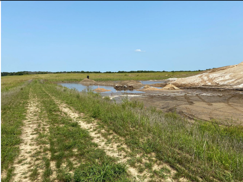
Photograph 12: View showing standing contact water between the soil berm and ash in Cell 1A.
