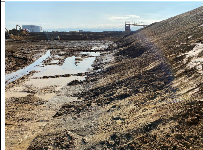
Photograph 8: #E View of the soft, wet areas at the toe of splitter dike separating the East Bottom Ash Pond and East Wastewater Pond.
