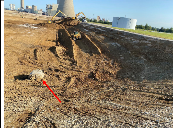
Photograph 7: #E View the interior slope of the EBAP, the plugged and partially demolished low level discharge structure noted by the red arrow.
