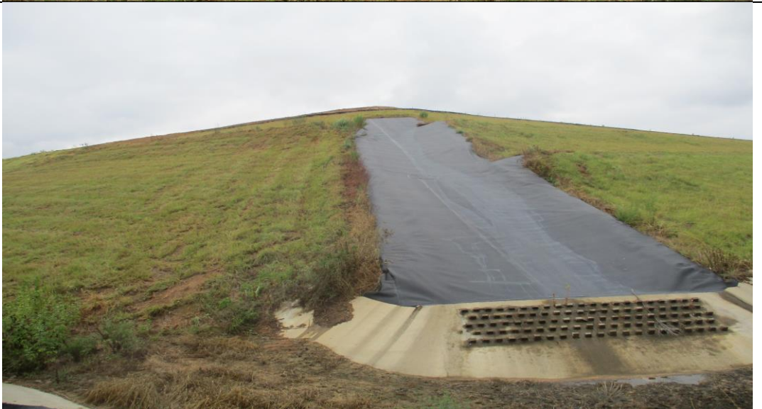
Photograph No. 3 View of the northeast corner let down to the ditch.
