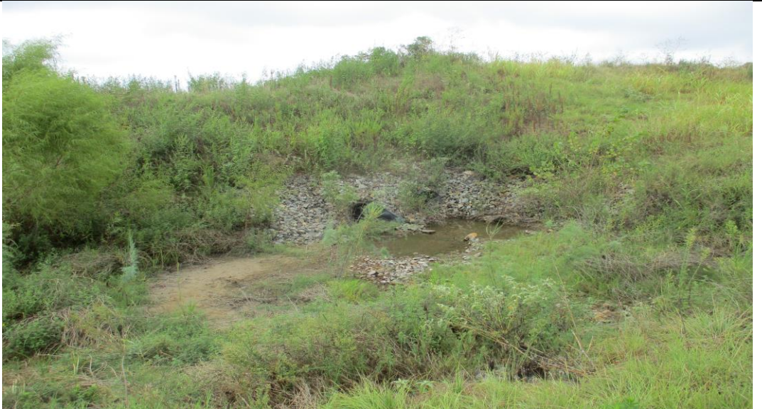
Photograph No. 10 Landfill runoff pipe culvert in the northwest area of the landfill.
