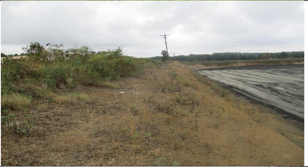
Photograph No. 11 View of the west dike interior southern section (looking north).
