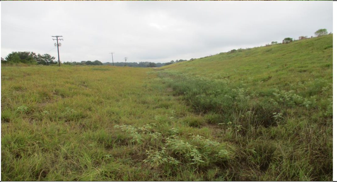
Photograph No. 8 Overall view of the north slope and the toe ditch (looking east).
