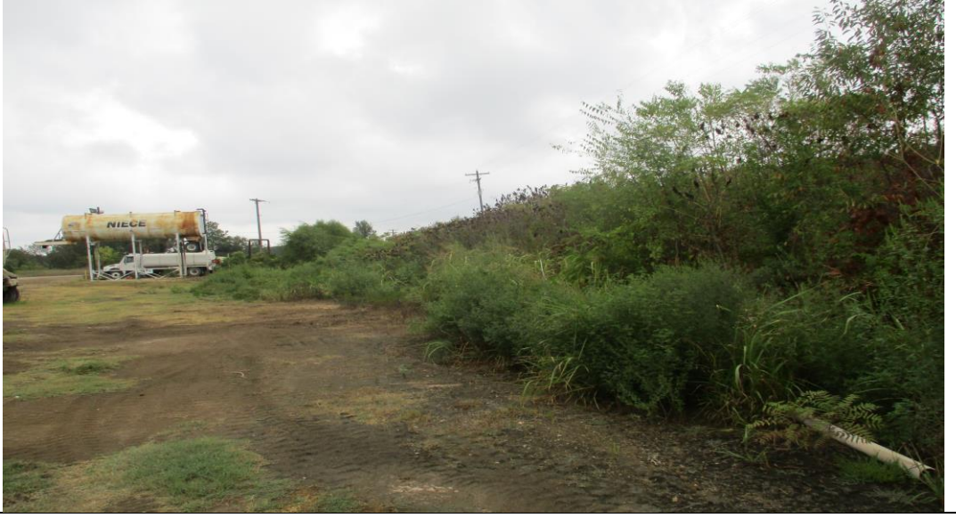
Photograph No. 12 Typical view of the west dike exterior slope (looking north).
