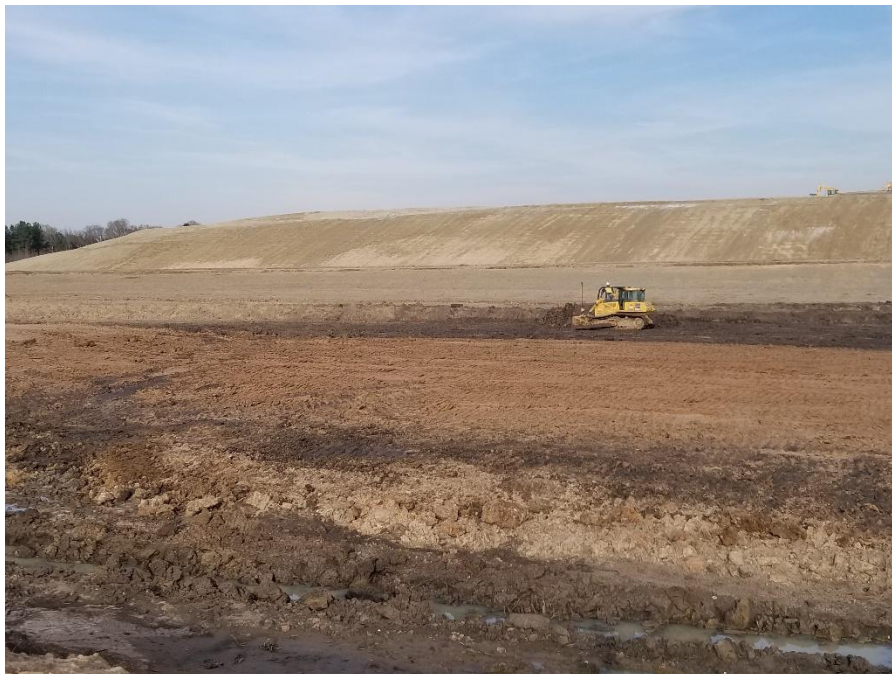
Looking east at dozer grading cell floor before placement of clay liner material.
