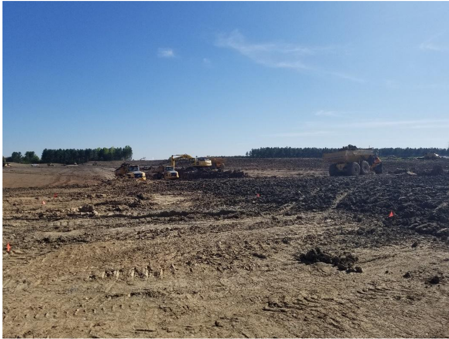
Looking south at excavators cutting structural fill material and loading into haulers to be transported.
