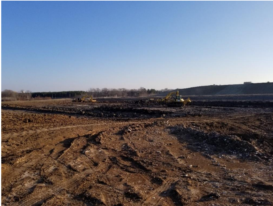
Looking northeast at Excavators cutting overburden and loading into haulers to be used as structural fill.
