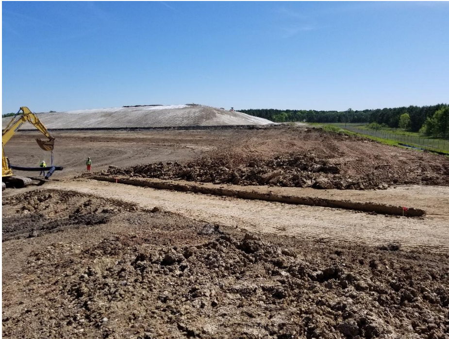
Looking east at excavators moving south leachate line to place in berm.
