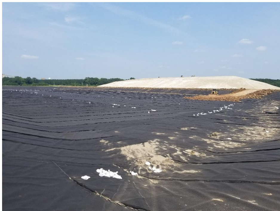
Looking northeast at dozer beginning to spread protective cover material into cell floor.
