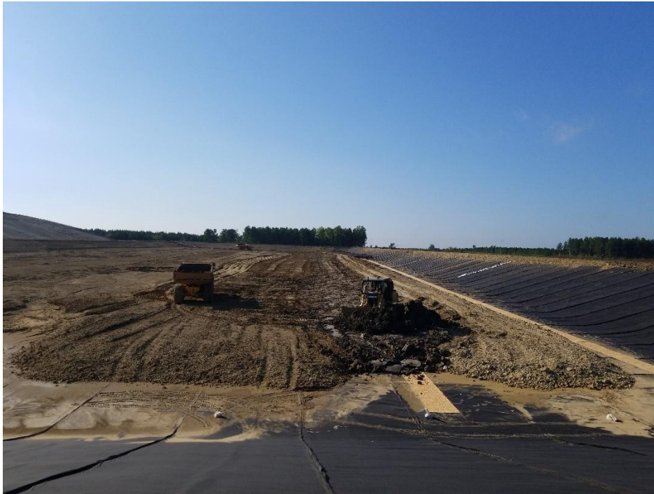
Looking south at placement of protective cover material. Also shown is plywood placed for protection of geosynthetics for future chimney drain and leachate line trench excavation.
