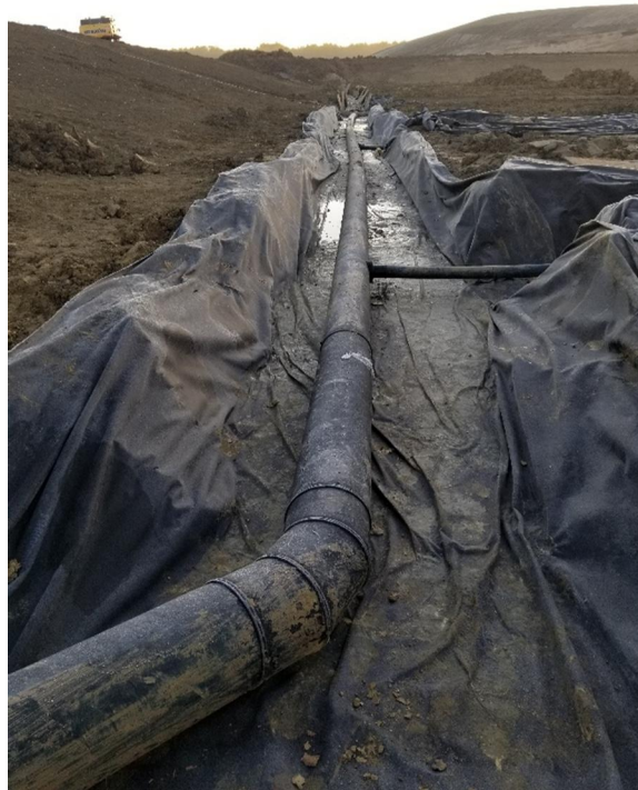
Looking east at north leachate line connections.
