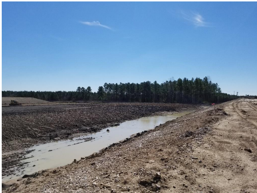
Looking southeast at ponded material outside beginnings of west berm after a heavy rain.
