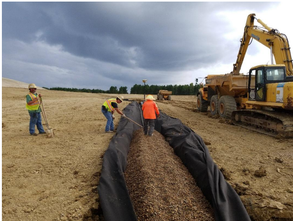
Looking at placement of gravel in leachate trench, and surveyor verifying gravel thickness.
