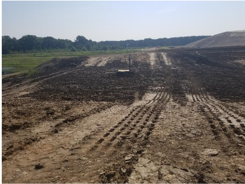
Looking east at manhole in north berm after placing material above leachate line.
