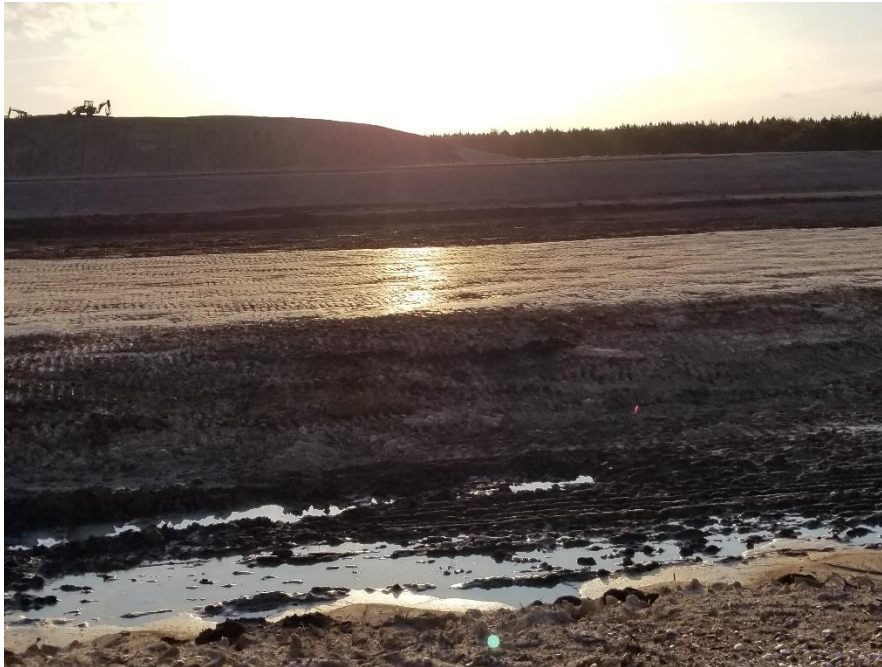
Looking east at west berm after smooth drum sealed it to prevent moisture infiltration.
