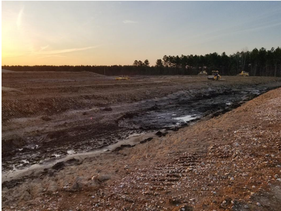
Looking southeast at smooth drum roller left in place after creating density testing pads following clay liner placement.
