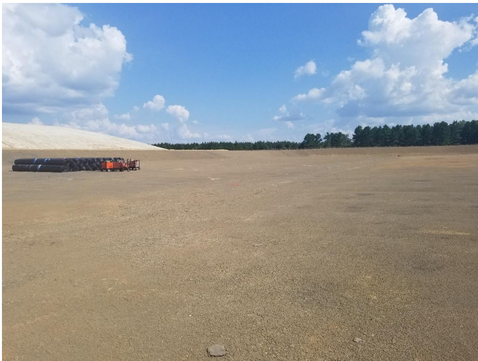
Looking south at completed clay liner and geomembrane being staged prior to deployment.
