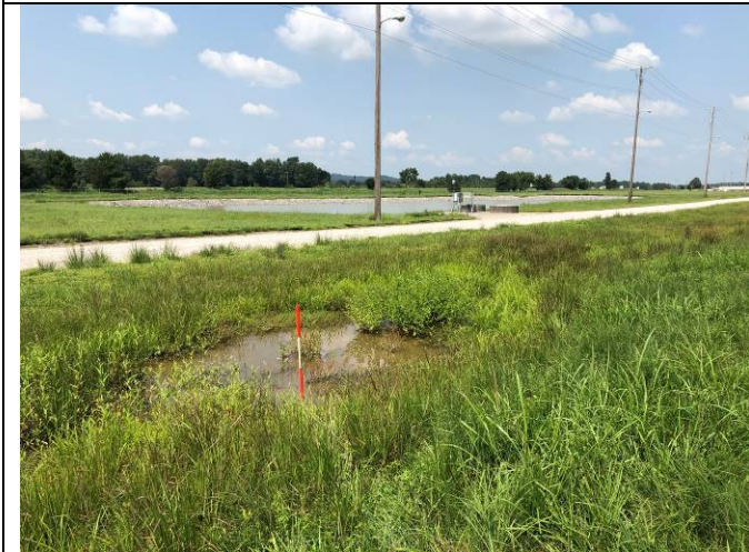
Photograph 2: #W View of standing water noted beyond to the toe of the embankment dike of the west bottom ash pond.
