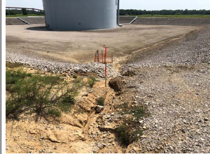
Photograph 7: View of erosion rill on the northern groin between the metal cleaning tank containment dike and the east bottom ash pond dike.
