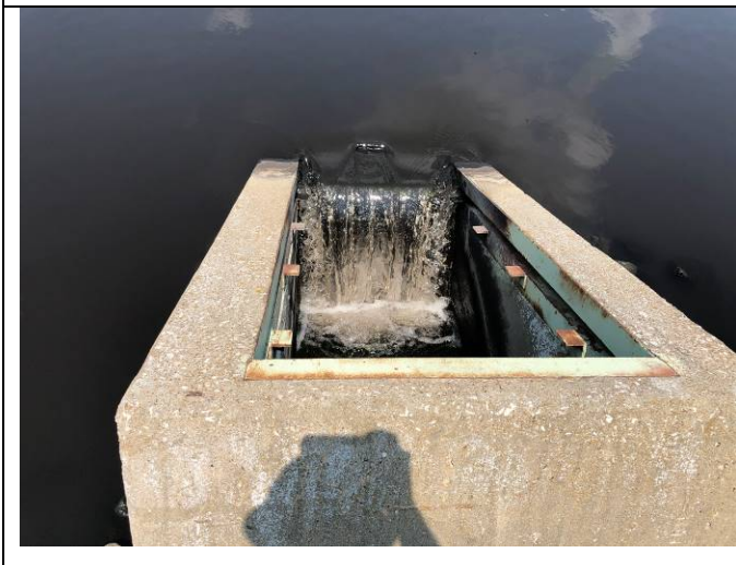
Photograph 3: #W View of the low-level discharge structure at the west bottom ash pond.
