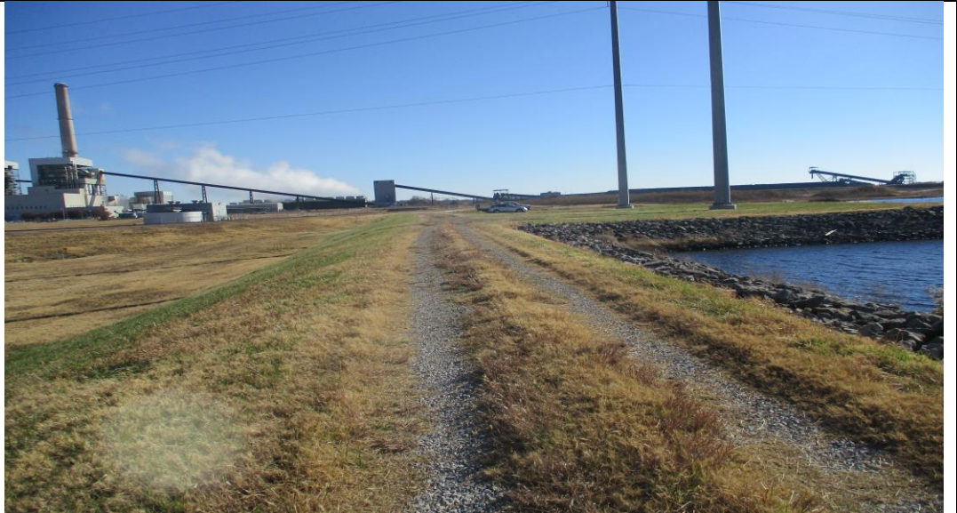
Photograph No. 4 Typical condition of the crest of the northwest dike section (looking east).
