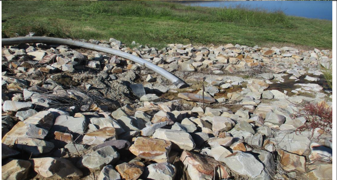
Photograph No. 23 Cell 2 leachate pipe outlet.
