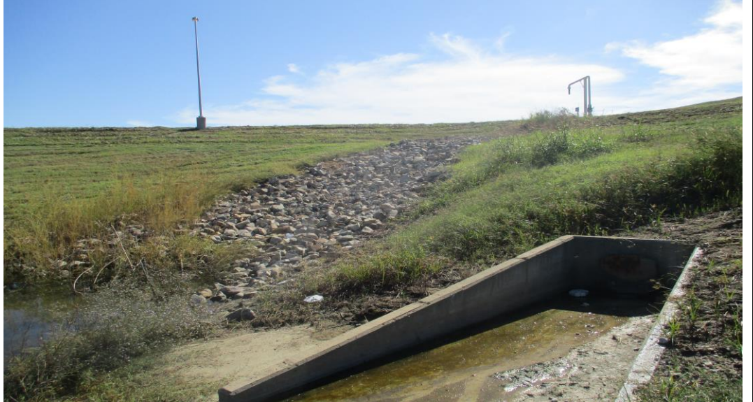
Photograph No. 22 Cell 1 leachate pipe outlet.
