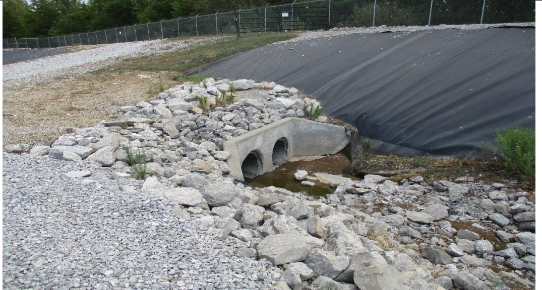
Photograph No. 17 Leachate pond south side perimeter runoff channel and pipe culvert outlet (looking east).
