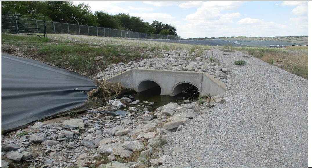
Photograph No. 16 Leachate pond south side perimeter runoff channel and pipe culvert outlet (looking west).
