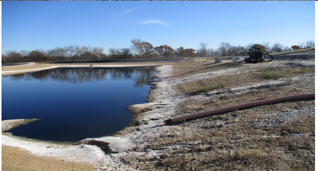
Photograph No. 20 Interior slope of the west dike, minor erosion.
