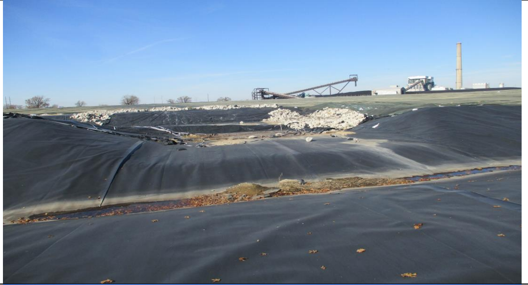
Photograph No. 8 Temporary stormwater control weir.
