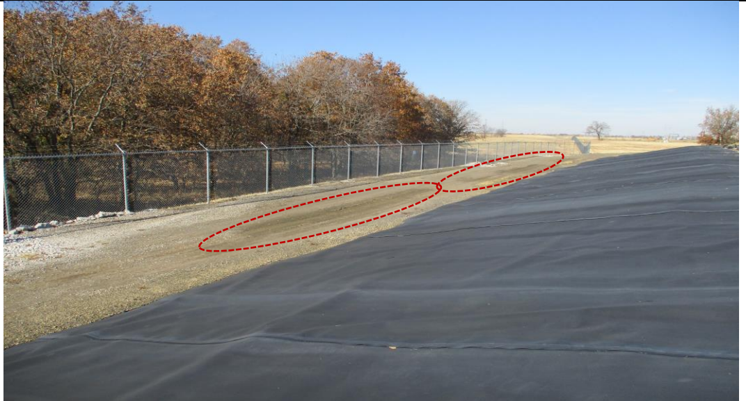
Photograph No. 4 Minor erosion at the access road.
